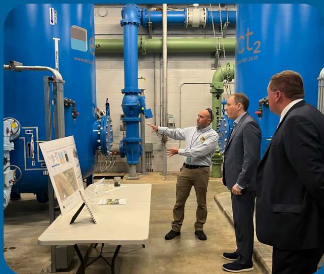
City of Portsmouth's Water Operations Manager, Tim Green, describing the ion exchange PFAS removal process to Administrator Zeldin.
