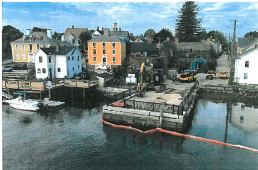
Photo 2: Similar viewpoint from photo 1, Overview of LaCava Wharf after August 2019 demolition, photo taken 8-30-2019.
