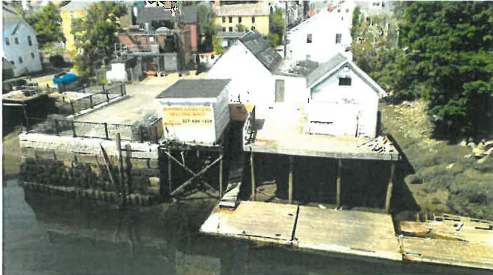
Photo 1: Overview LaCava Wharf before August demolition, photo taken 7-7-2014. Proposed floating docks will be placed in front of the visible seawall, next to the existing floating docks shown.
